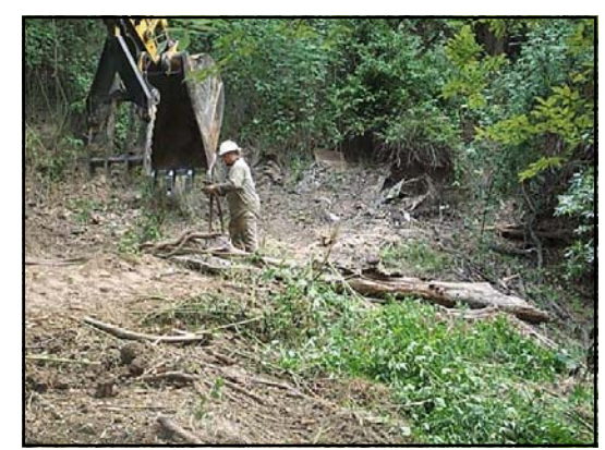
Debris removal is one of the cooperative projects that can be accomplished more efficiently under the BRWM partnership.
